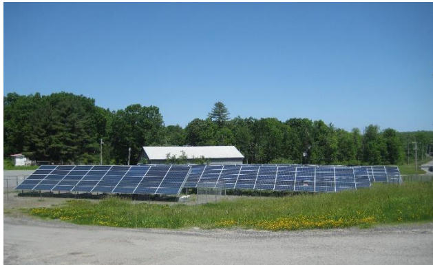
3.13. Solar Panels at Town Highway Department
